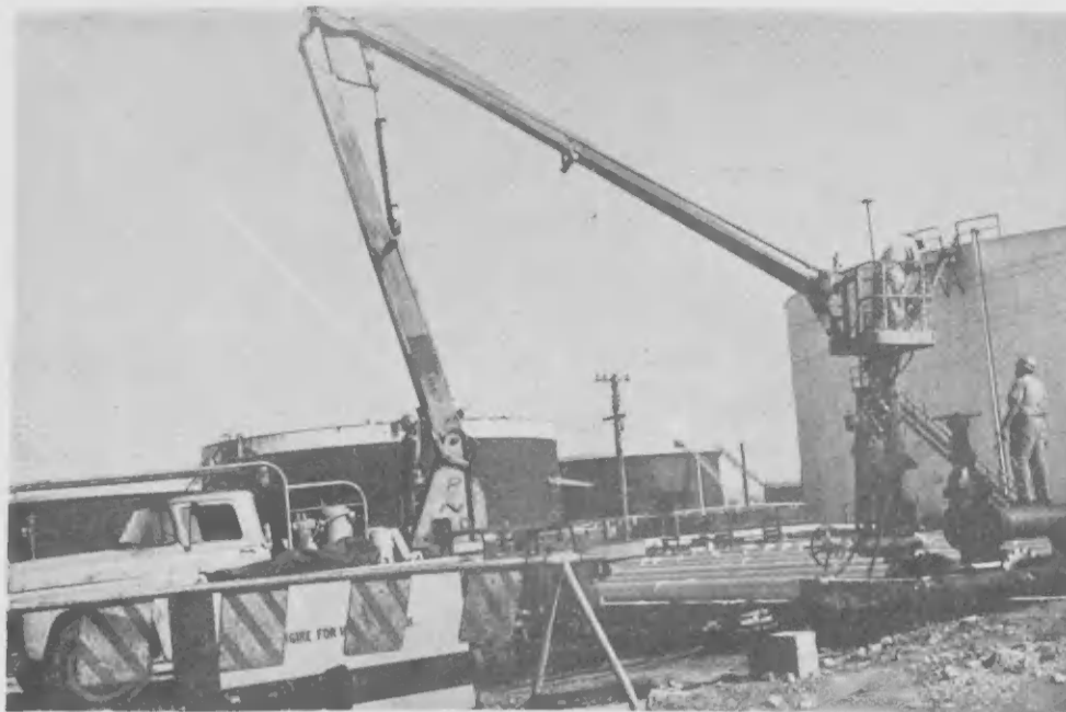
Giraffe's long neck is essential at some locations in pipe alleys. It enables the Mechanical men to make adjustments to tapping machine. Final arrangements and checks precede drilling operations. Inside view shows circular saw after cut is made.
